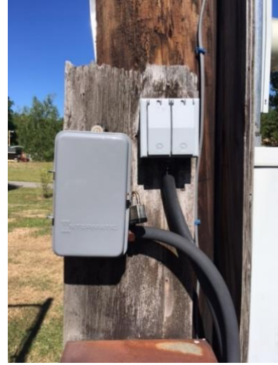
Timer box (locked) and light switches
