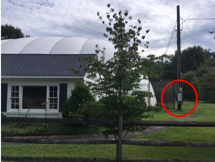
AITA clubhouse and light controls (circled).
